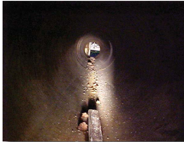
MPW's video inspection cameras provide an accurate account of the pipe's internal condition and cleanliness following a line pigging project.
