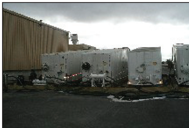
MPW frac tanks were used as part of a parallel wastewater treatment system, while plant personnel made necessary inspections and repairs to underground treatment systems.
